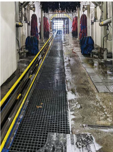
Track & Hydronic System
