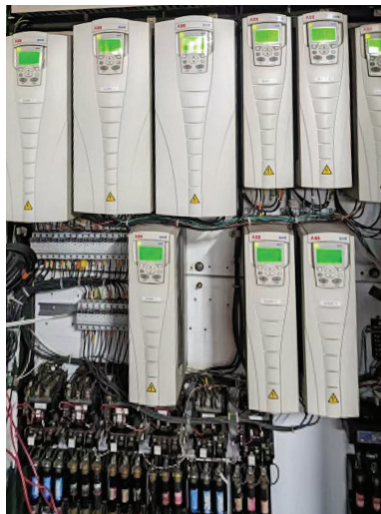
VFD Control System
